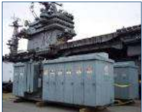
Mobile Utilities Support Equipment
